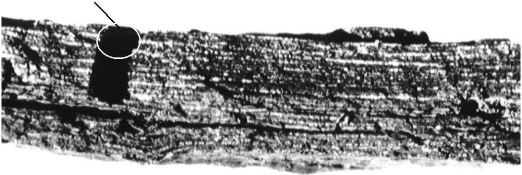
Fig. 5. Longitudinal section of the additional tunnel in front of the access/exit hole, showing the thin wall left by the larvae of Calydon submetallicum .
